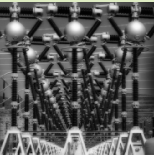
HEP's transmission system - a connection with the world
