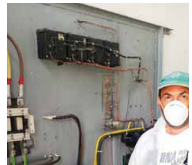
...energetskog transformatora u PTTS Velebit u Gunji...
