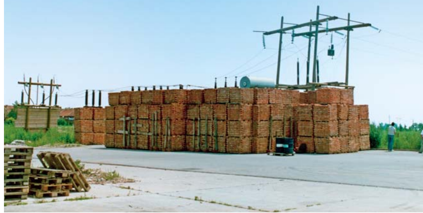
TS 110/35 kV "505", 22 MVA
