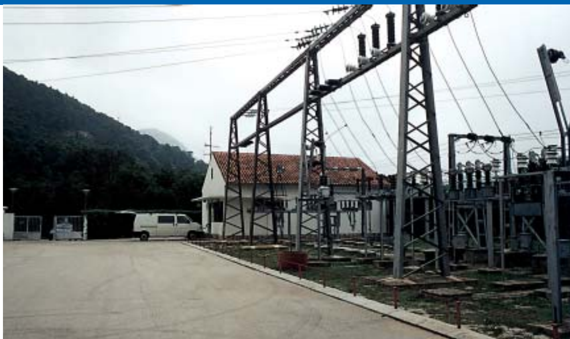
TS 110/35 kV Ston
